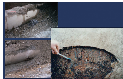
图1 传统金属材质管道结构腐蚀实物图 Fig.1 Corrosion photo of the traditional pipe made of metal and cement materials
