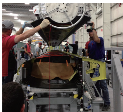
图5 V-280机翼制造: 蒙皮与肋胶接 Fig.5 Wing manufacturing of V-280: bonding between skin and ribs
